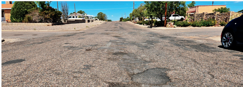
Marie Street road damage
