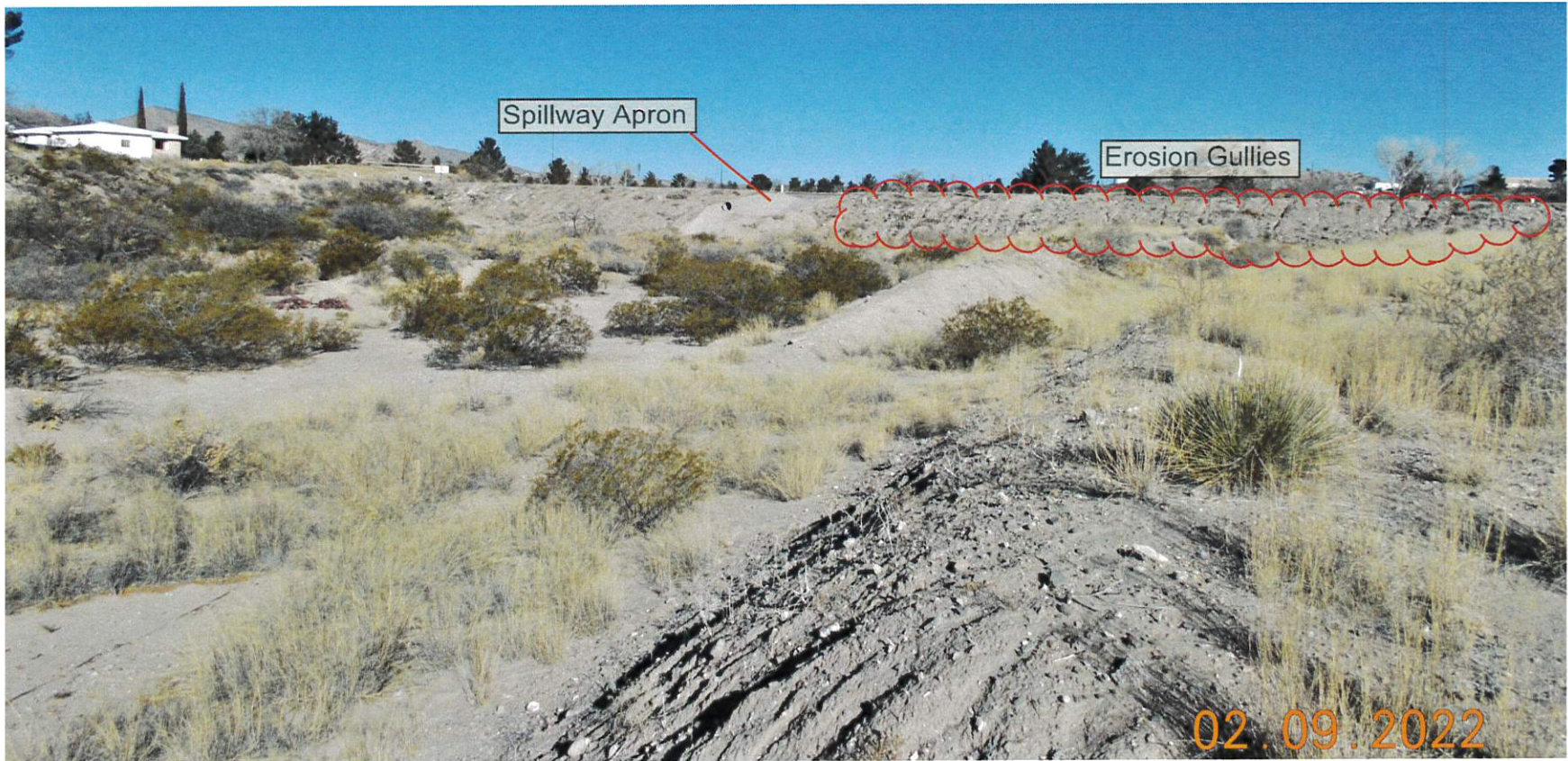
8. Image 8: Northerly view of the downstream slope with areas of erosion and spillway apron as indicated.
